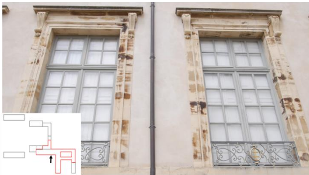
25 Figure S11: Photographs of the Lunéville château and their location on the sketch of the château (the zone in red represents the zone affected by the 2003 fire). Dark patinas affect only specific sandstones blocks.
